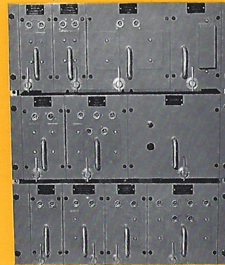
Electronic systems rack
